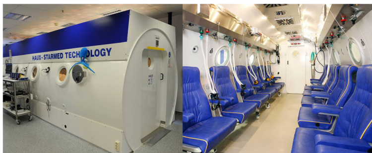
Figure 1 Exterior and interior view on the pressure chamber for max. 12 persons.
